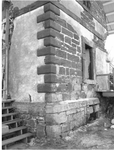
The conservation team focused primarily on the northeast corner of the ruin
