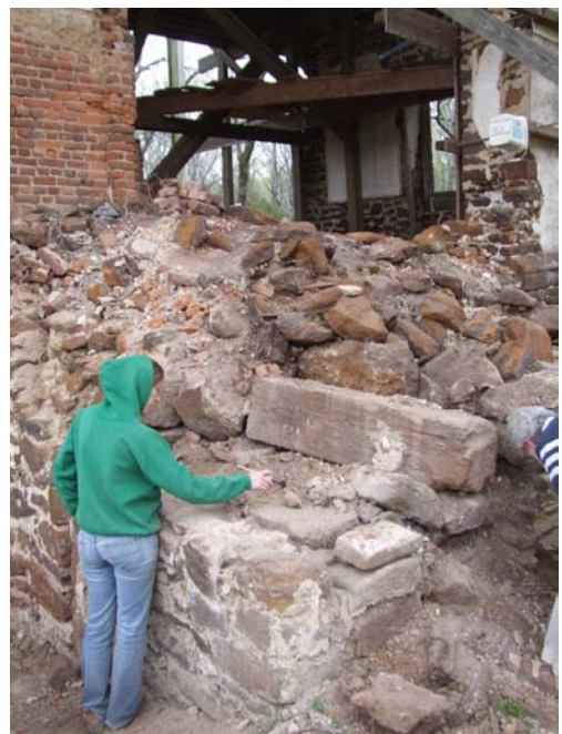
Locating the Door jamb in the rubble
